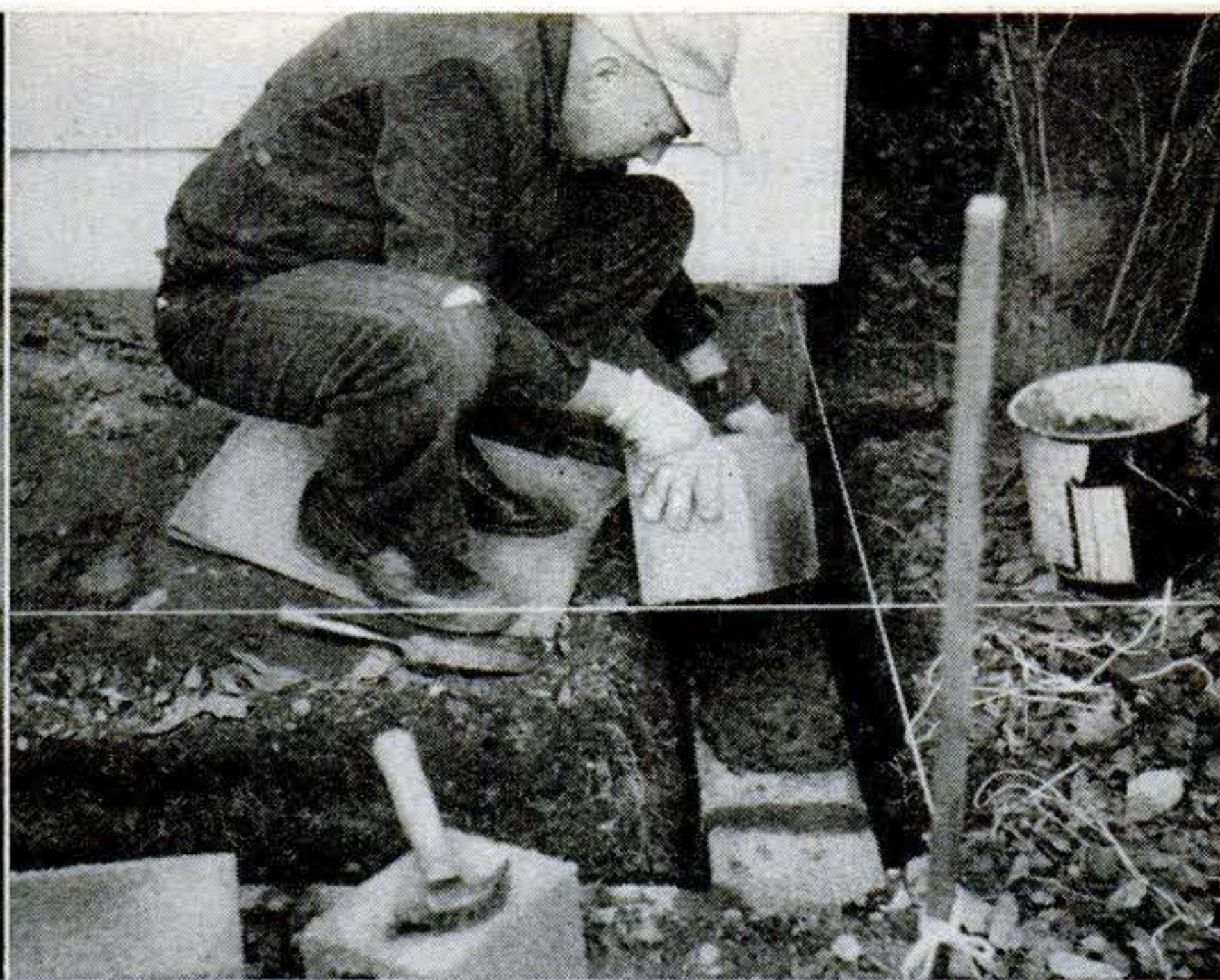
2 CINDER BLOCKS are laid on top of footing. Staked cords, carefully leveled, help to align blocks vertically and horizontally. I built sides one course higher than back.
